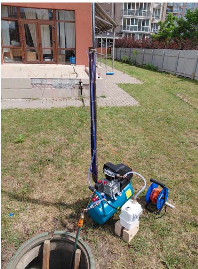
Fig. 3. Photo of an experimental installation for injecting air into a low-pressure aquifer
